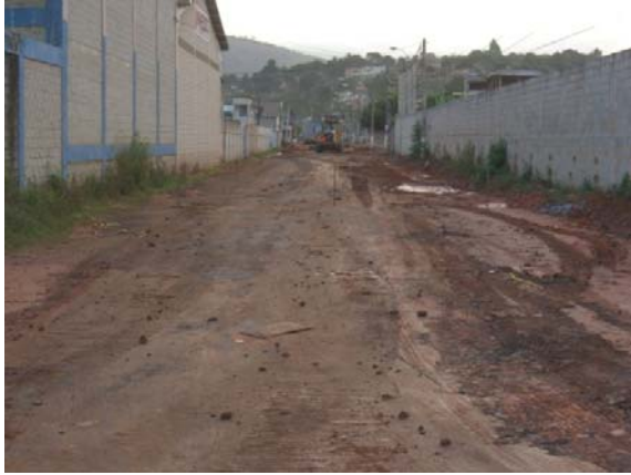
Figure 7. Regularization of the subgrade for the installation of geotextile [GTW] and geogrid [GG].
